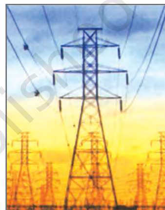
Fig. 3.7: National Power Grid to supply Electricity
