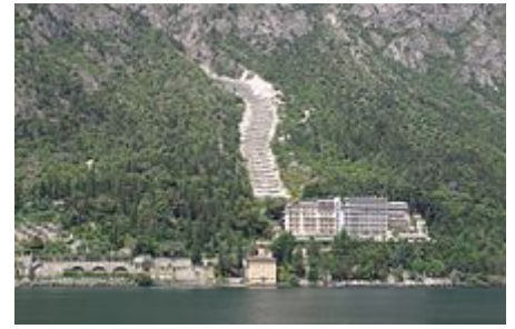
Hotel Panorama at Lake Garda. Part of a hill of Devonian shale was removed to make the road, forming a dip-slope. The upper block detached along a bedding plane and is sliding down the hill, forming a jumbled pile of rock at the toe of the slide.
