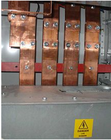
Copper electrical busbars distributing power to a large building
