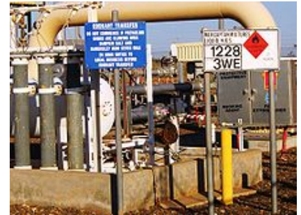
A pipeline odorant injection station
