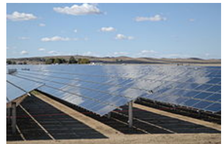
Solar panels at the 550 MW Topaz Solar Farm
