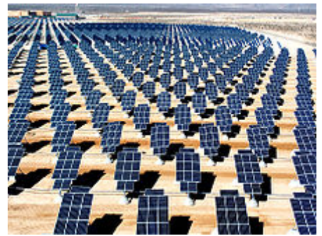
Nellis Solar Power Plant photovoltaic power plant in Nevada, USA
