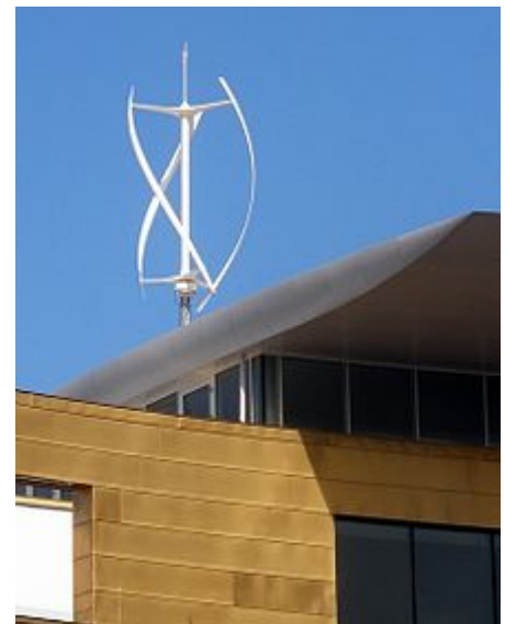
A small Quietrevolution QR5Gorlov type vertical axis wind turbine on the roof of Colston Hall in Bristol, England. Measuring 3 m in diameter and 5 m high, it has a nameplate rating of 6.5 kW.
