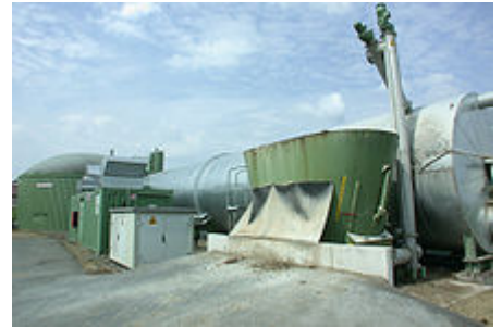
Pipes carrying biogas (foreground) and condensate
