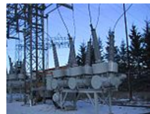
A high-voltage circuit-breaker employing sulfur hexafluoride SF 6 as its inert (air replacement) interrupting medium. [115]
