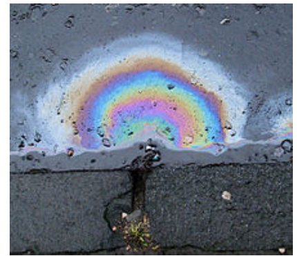
Diesel fuel spill on a road.
