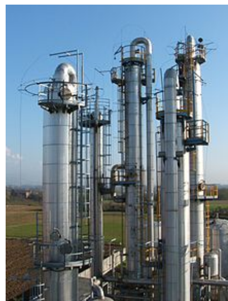
Typical industrial distillation towers
