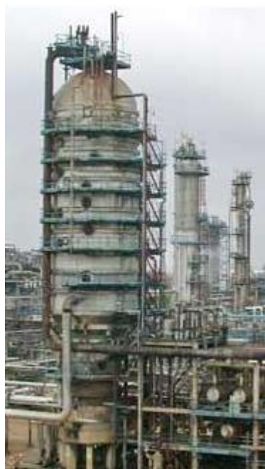
Large-scale, industrial vacuum distillation column [36]
